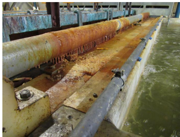
Figure H-7. Buildup of Chemicals Occurs Between Tanks Due to Lack of Drip/Drain Board
