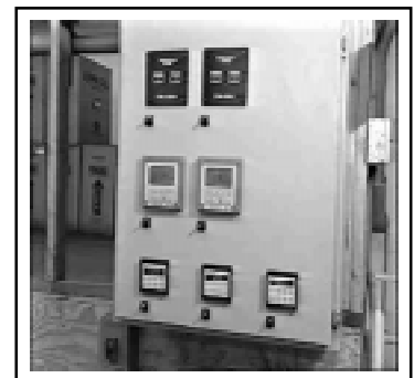
Figure 6. Analyzer Panel at the Artistic Facility
