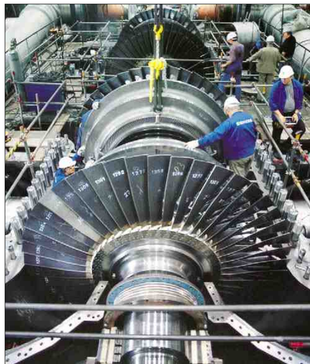
Figure 3 —Siemens power turbine assembly with the case open, clearly showing the significant size of the turbine blades (Photo: Wikimedia Commons, 2005; http://creativecommons.org/licenses/by-sa/3.0/ ).
